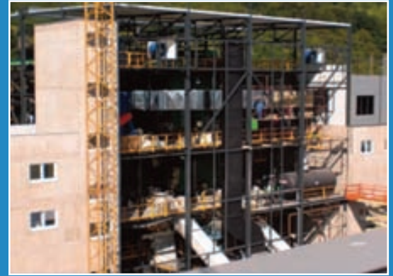
Turn-key project handed over by Urbas: The biomass fired co-generation power station in the town of Bardejov in East Slovakia.
