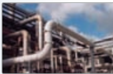
Piping & Fire Protection
